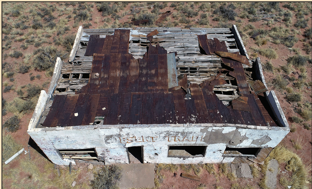
The building's roof sagged from decades of unchecked wind, rain and snow.
